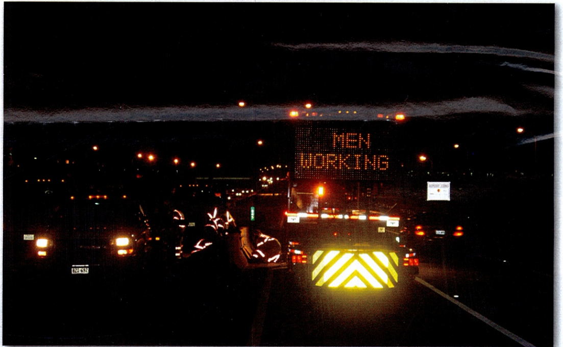
LED DoT lighting is built into the MBT-1 Mobile Barriers Trailer, providing a safe work environment at night.
