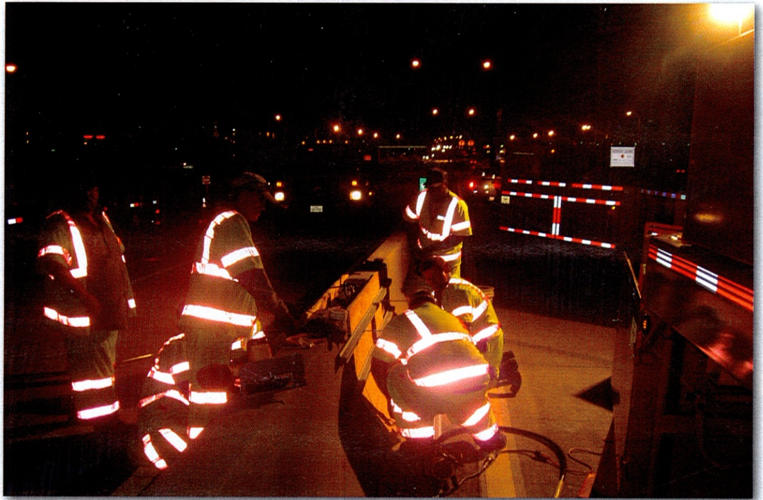
Workers are kept safe while repairing a barrier in the protected work zone provided by the North Texas Tollway Authority's MBT-1 Mobile Barriers Trailer.
